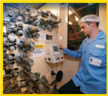
In a difficult lacquer handling application, close coupled pumps saved time and money
