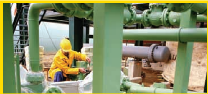
In an aggressive chemical recovery application, the pump paid for itself in less than 12 months
