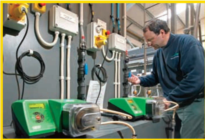
500 series pumps replaced troublesome diaphragm pumps for coagulant dosing
