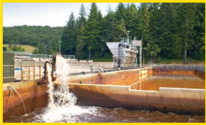
At a remote water treatment works, chemicals are metered to balance pH levels
